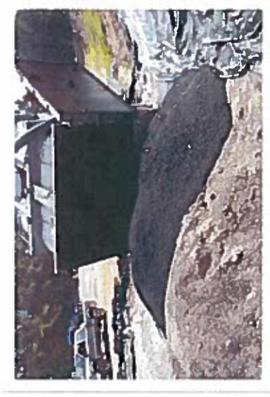
Piles of Dumped Spoils
